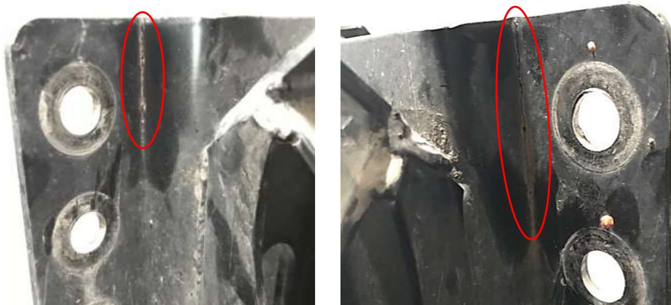
Figure 3. Cracks (circled) at bracket bend lines.
