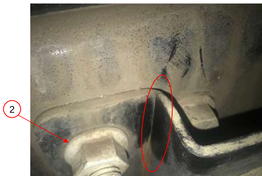
Figure 2. Crack at front bracket corner bend (circled) adjacent to mounting bolt (2).
