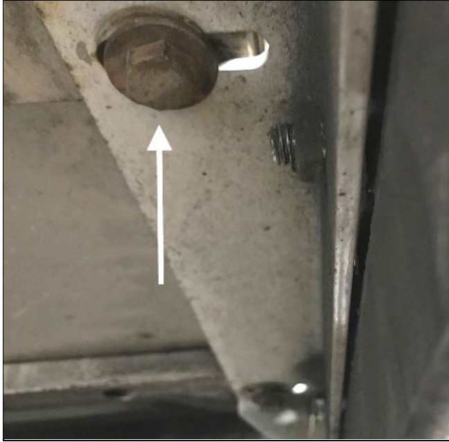
FIGURE 14: BATTERY TRAY BOLT (3X UNDERSIDE)
