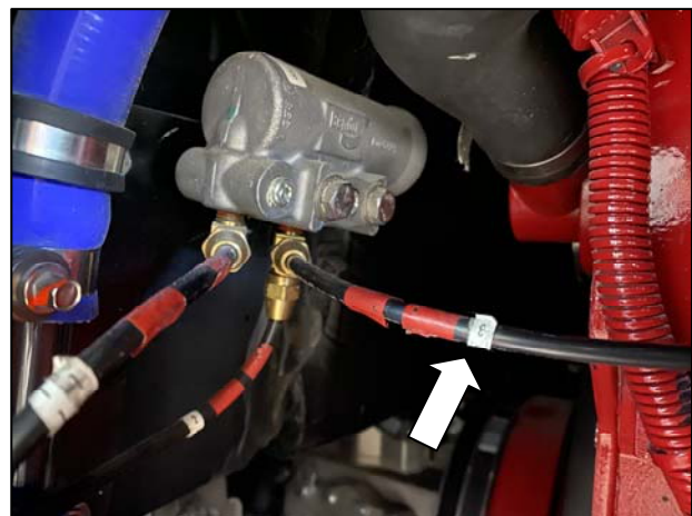
Figure 2: Affected compressed-air line at governor side
