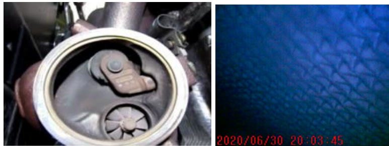
Figure 4 - turbo shaft from catalyst side and inside the catalyst
