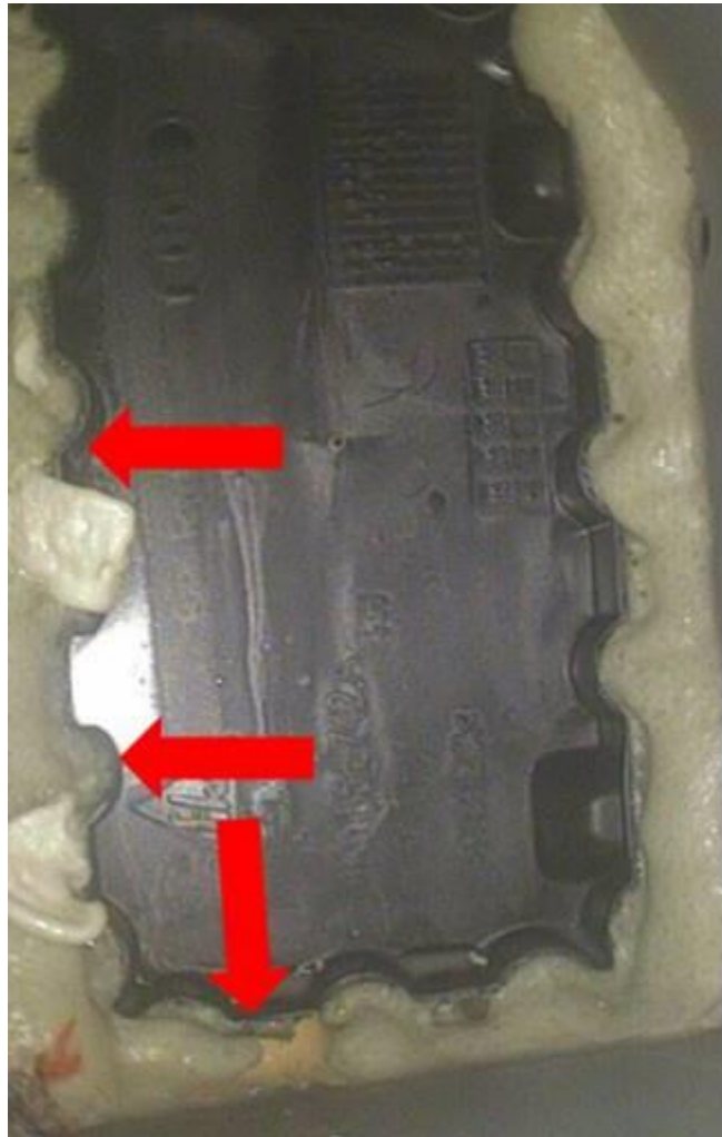
Figure 1. The exact location of the water intrusion.
