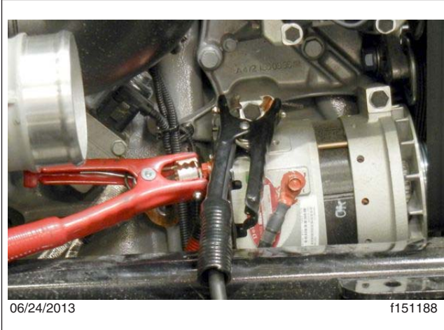
Fig. 7, For EPA10 and EPA04 engines, the starter path can be checked by loading the circuit at the alternator.
