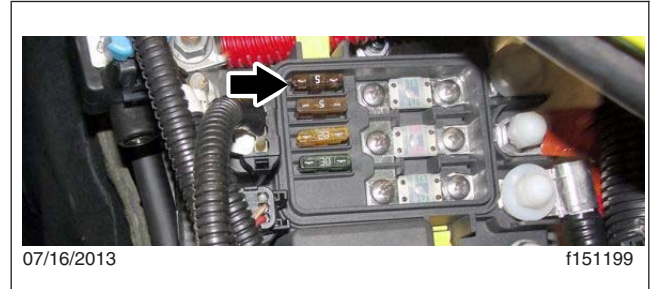
Fig. 15, EPA10 vehicles: 5 amp remote sense fuse, location D in the Powernet Distribution Box (PNDB).
