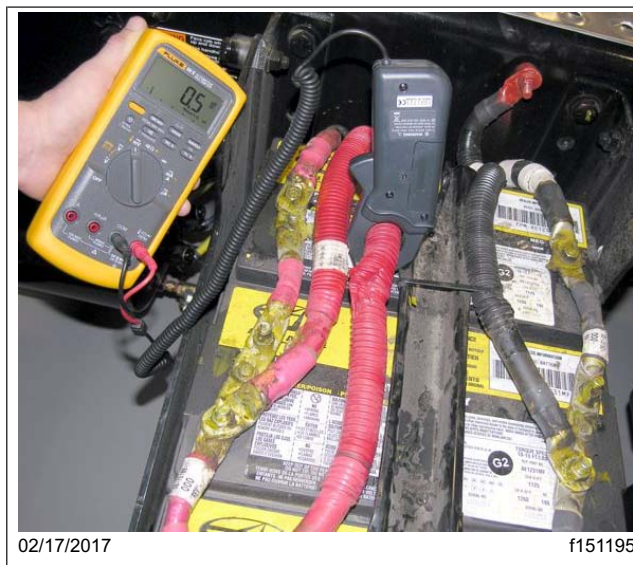
Fig. 12, After zeroing the amp clamp away from the vehicle, measure the amperage in each positive cable leaving the battery pack.
