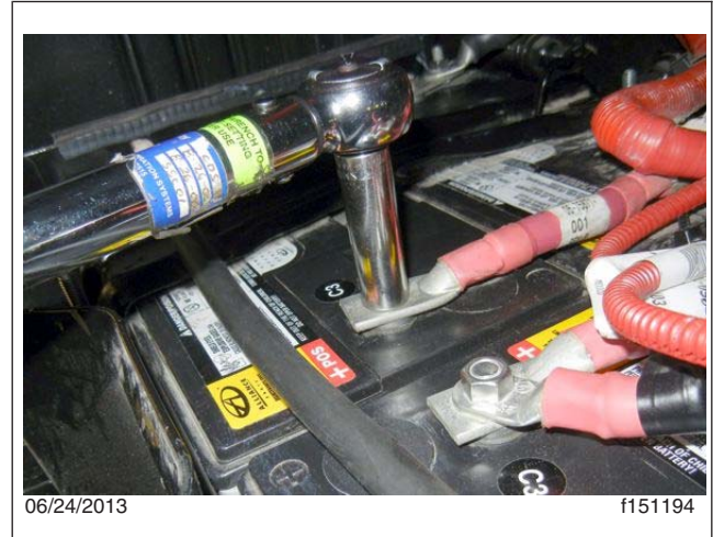
Fig. 11, Check the battery connections for looseness and corrosion. Check the torque on the connections.
