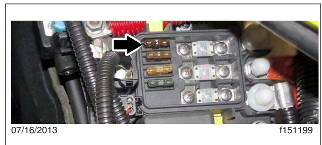
Fig. 15, EPA10 vehicles: 5 amp remote sense fuse, location D in the Powernet Distribution Box (PNDB).
