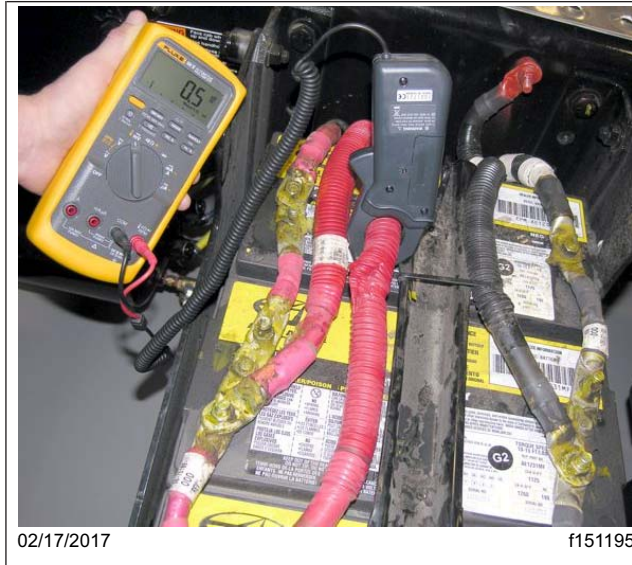
Fig. 12, After zeroing the amp clamp away from the vehicle, measure the amperage in each positive cable leaving the battery pack.
