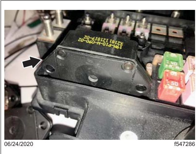
Fig. 1, High-Current Circuit Breaker in the BCA Box
