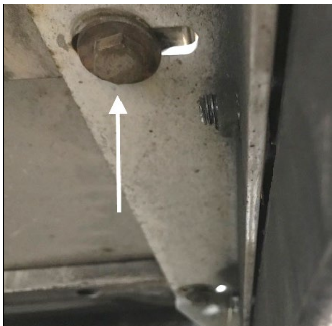
FIGURE 14: BATTERY TRAY BOLT (3X UNDERSIDE)
