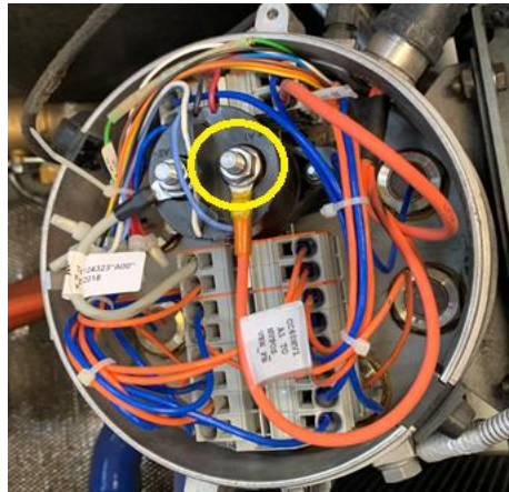
Figure 21: High Voltage Positive Auxiliary Heater Connection
