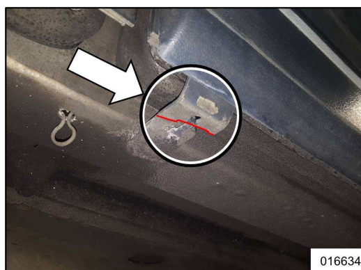
Figure 2: Typical break of the aluminium door lip
