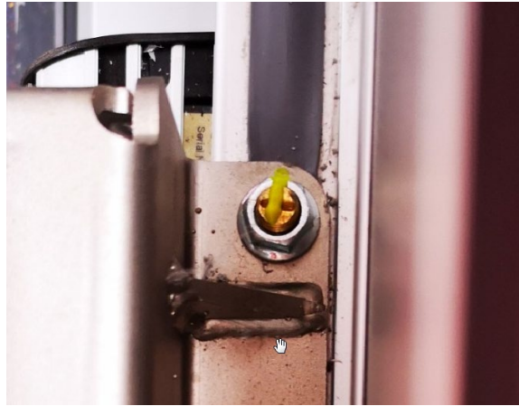
Example of T-bolt with top puncture facing the center of the bus
