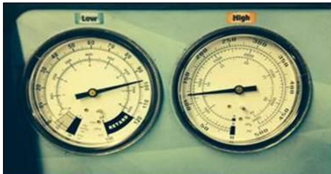
Figure 6. Equalized pressure condition. No pressure generated from compressor.
