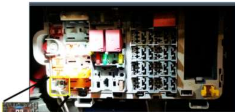
Fuse F82 (20 Amp JCASE Fuse) Located in the Rear PDC was Open/Blown
