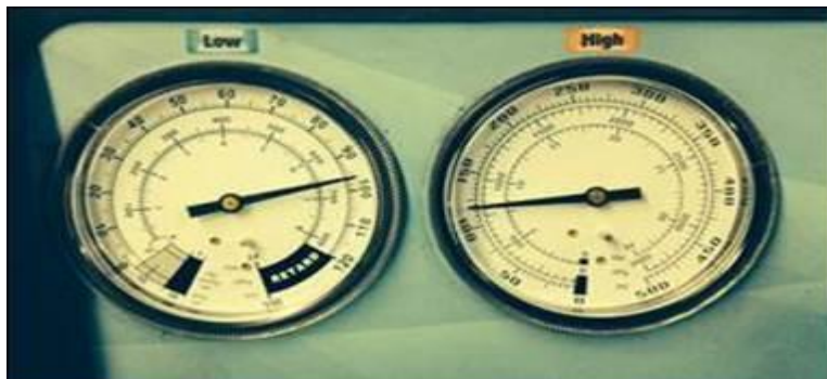
Figure 4. Equalized pressure condition. No pressure generated from compressor.
