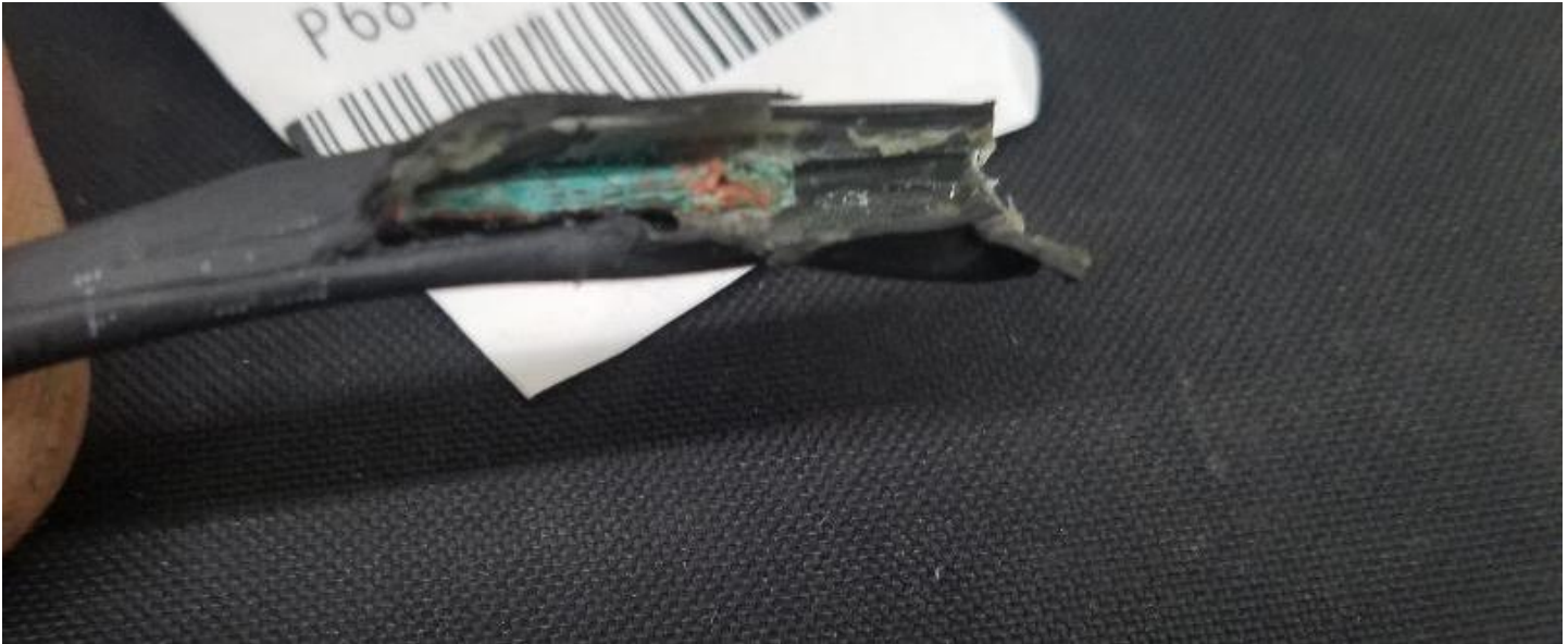
Corroded Splice SD403
