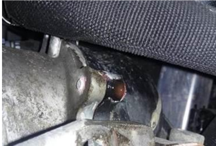
Figure 5. Coolant marks on coolant connector union.
