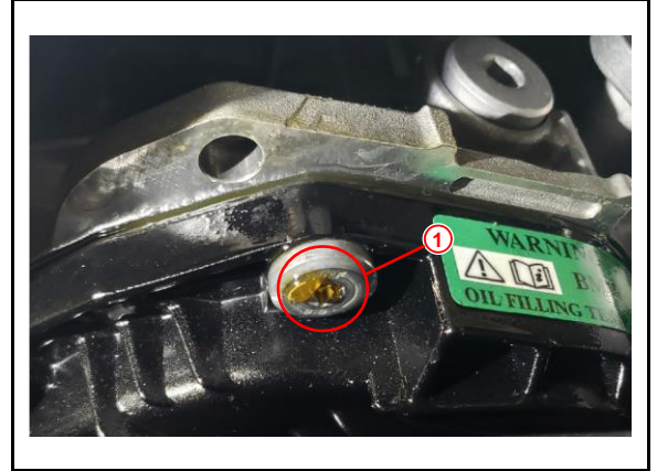
Figure 2. Oil Leak From Transmission Oil Pan
