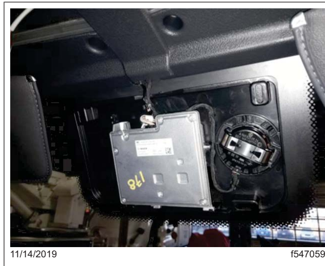
Fig. 5, Rain/Light Sensor Installed
