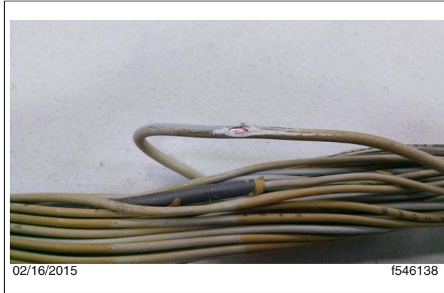
Fig. 1, Worn Insulation, Major
