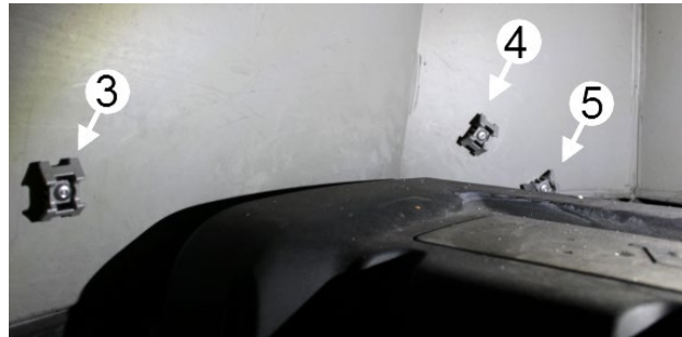
FIGURE 110: TIE MOUNT 3 & 4 SHALL NOT BE PLACED BETWEEN THE BULKHEAD AND THE VALVE COVER.
