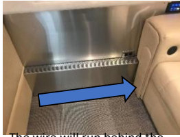
The wire will run behind the convactor closeout. The wire should rest at the bottom of the cover and not on top of the convectors.
