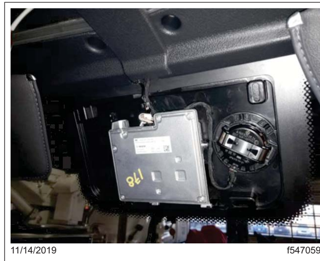
Fig. 5, Rain/Light Sensor Installed
