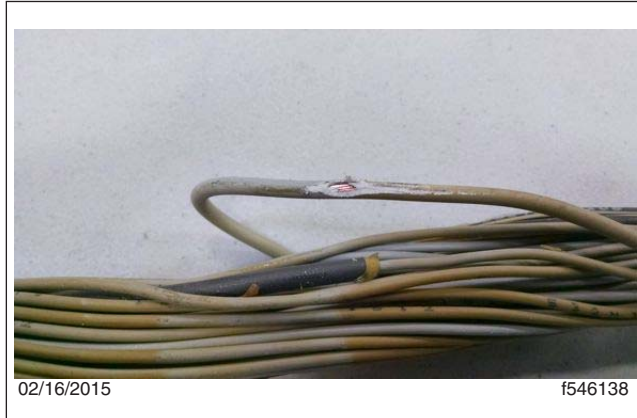
Fig. 1, Worn Insulation, Major
