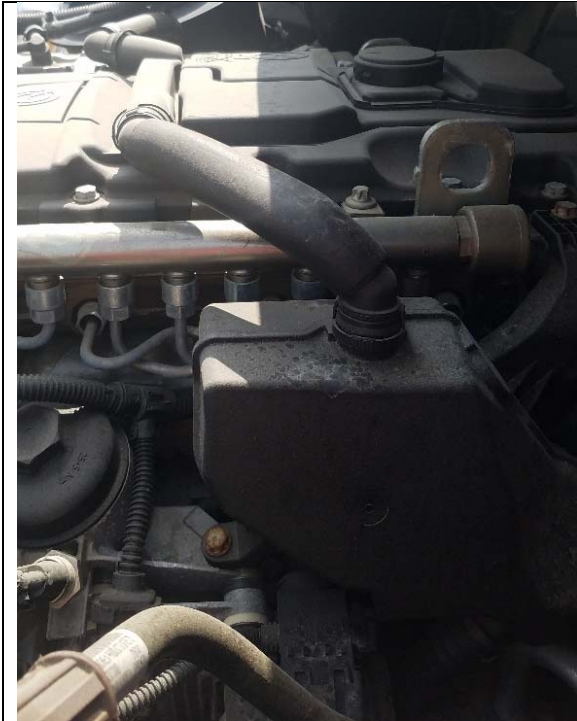
Original Air Compressor Upper Suction Line
