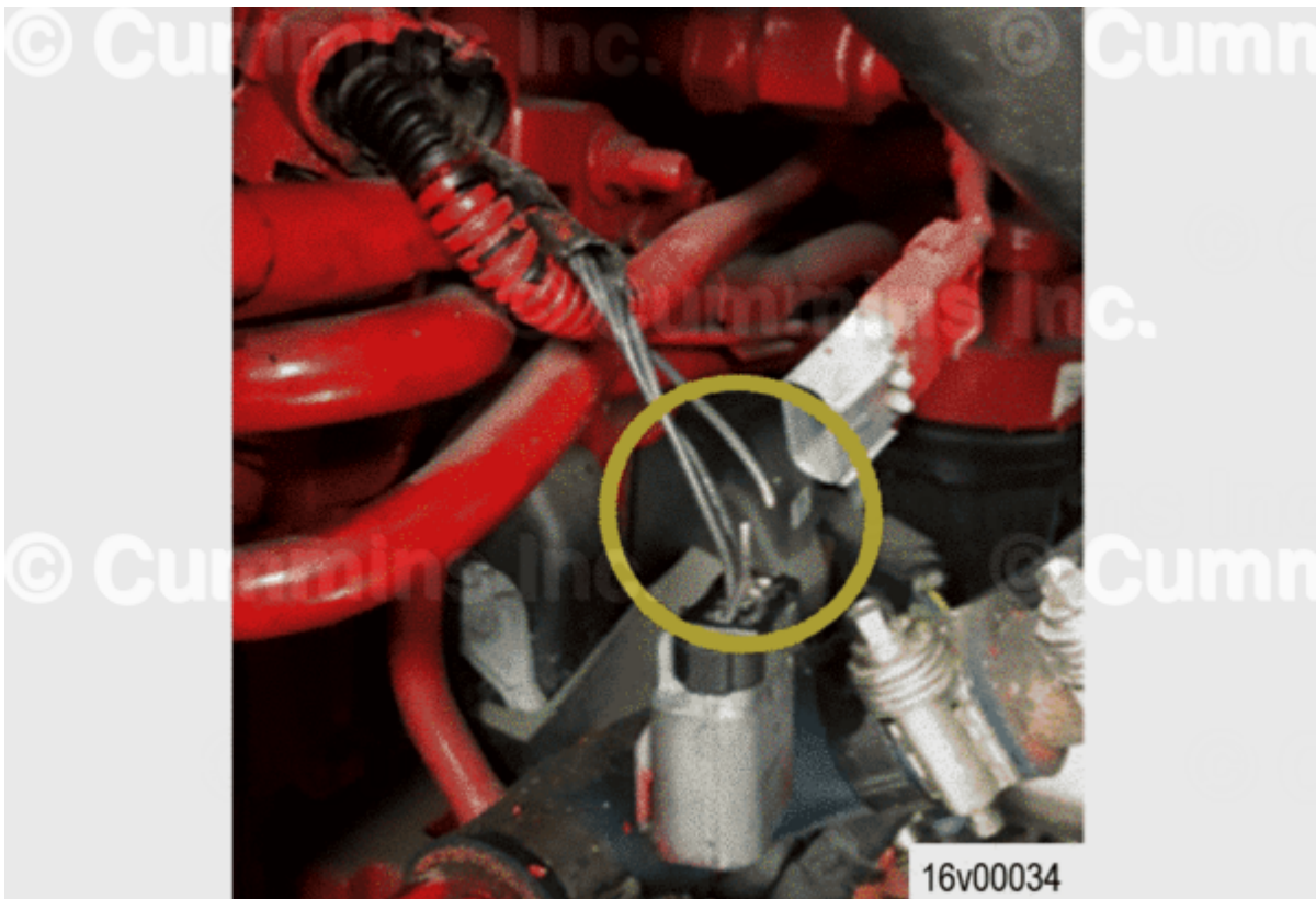
Figure 2, Example of Damaged Wiring.
