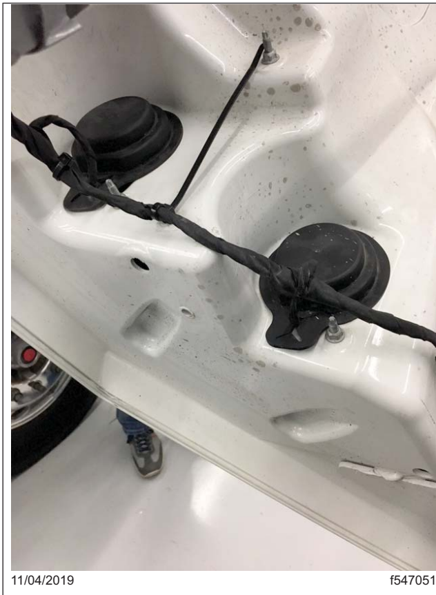
Fig. 9, Lamp Cavity Covers Properly Installed
