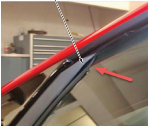
OUTER DOOR SEAL GAP
