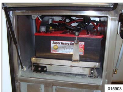
Figure 1: Battery compartment in front of RH drive axle wheels (batteries mounted in longitudinal direction)
