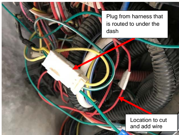
Figure 4: Plugs Behind the PC Boards
