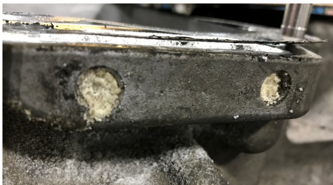
Clogged vent ports
