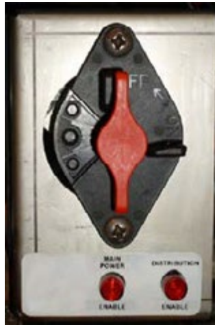
Figure 1 - Battery Disconnect Switch
