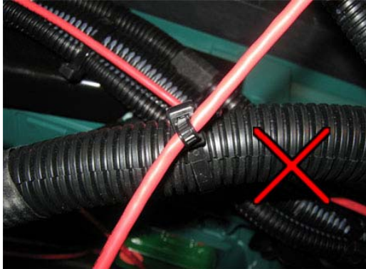
LTD extending slantingly from the cable tie
