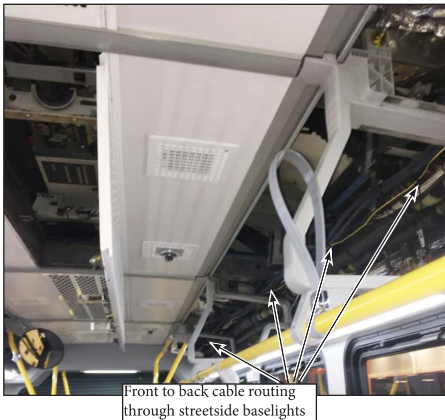
Figure 22 - Front to Back Cable Routing in the Streetside Baselights
