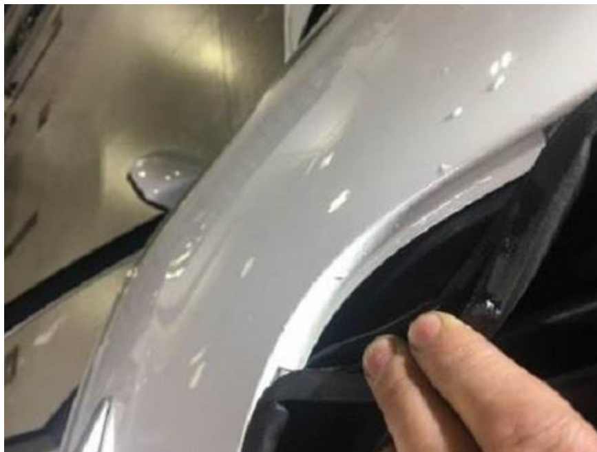
Figure 2: Example of the sunroof body side seal not having proper adhesion to the body.
