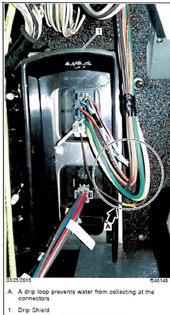
Fig. 1, SAM Chassis with a Drip Shield and a Drip Loop
