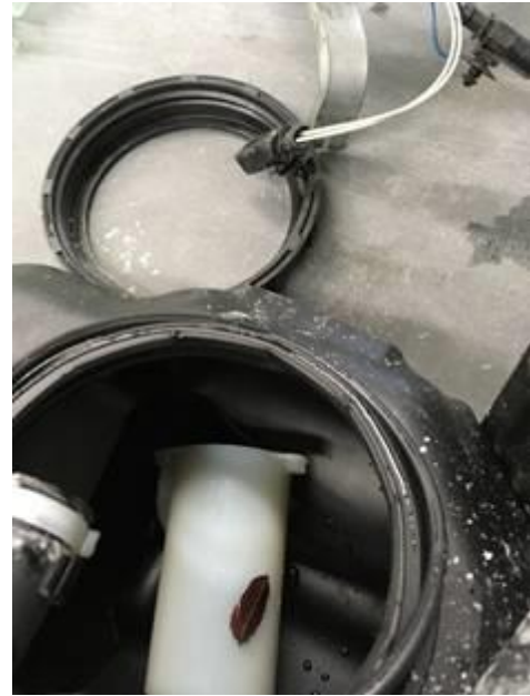
Figure 2. Filter element housing is loose inside the tank.
