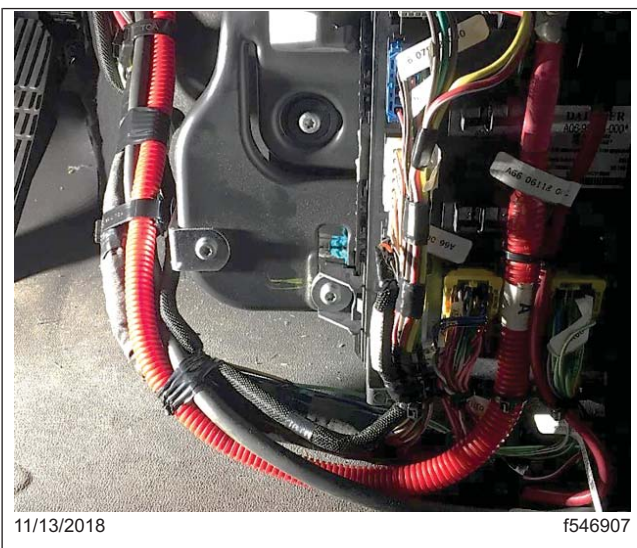
Fig. 6, Diode Routed and Wrapped with Electrical Tape
