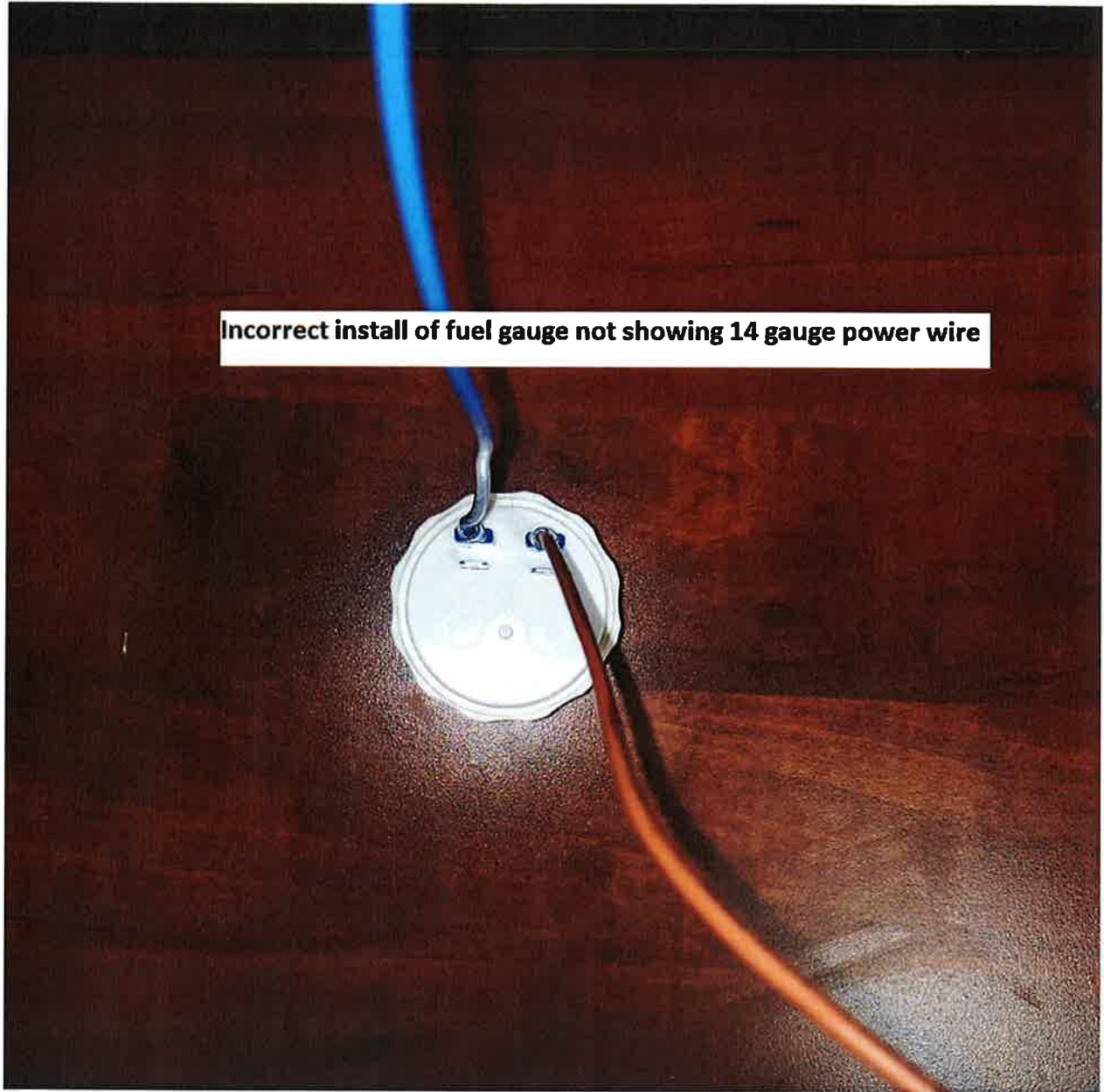
Pic 4. Incorrect wiring of fuel gauge
