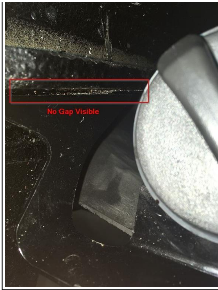
Figure 7 - Unacceptable Fill Receiver Bracket Gap
