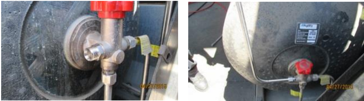
Figure 4. Left: Straight fitting mounted on cylinder valve. Right: Temporary L-shaped vent tube in place to vent gas up and out.
