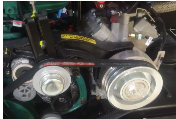
FIGURE 67: RUNNING HVAC SYSTEM
