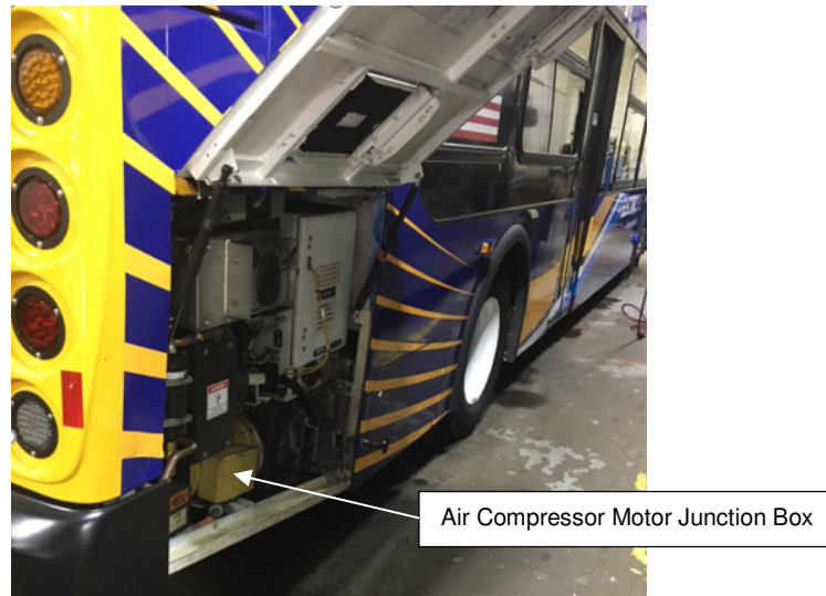
Figure 2: Air Compressor Motor Junction Box Location.
