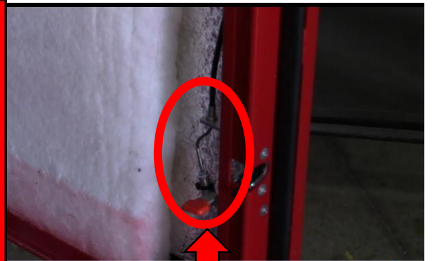
Incorrect Cable Adjustment
