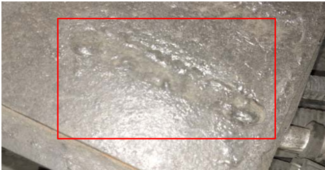
Poor Weld: Not completely filling slot
