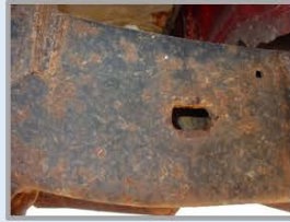
Light to Moderate Surface Rust
