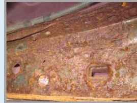
Complete Surface Rust with Descaling
