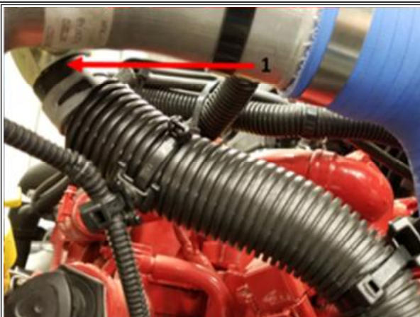
Figure 6: Air Compressor Inlet Hose
