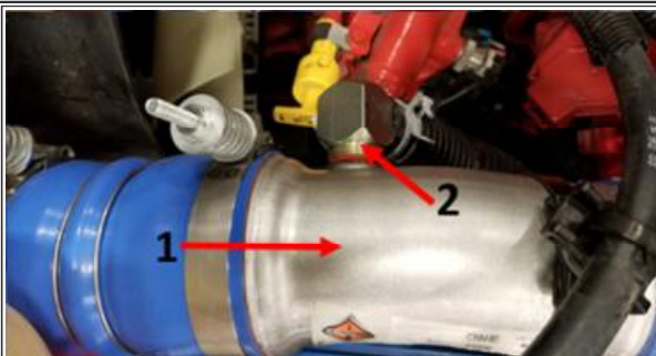
Figure 3: New charge air piping
