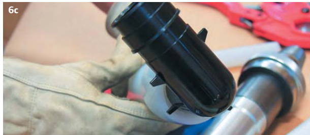
Insert ProPEX Fitting into 2" Uponor PEX Piping.
