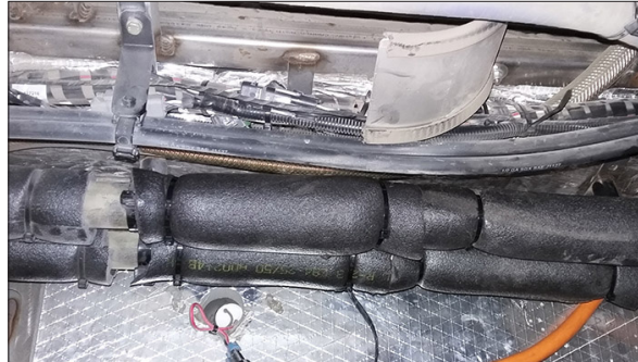
Figure 17 - Insulation on the Copper Pipes
