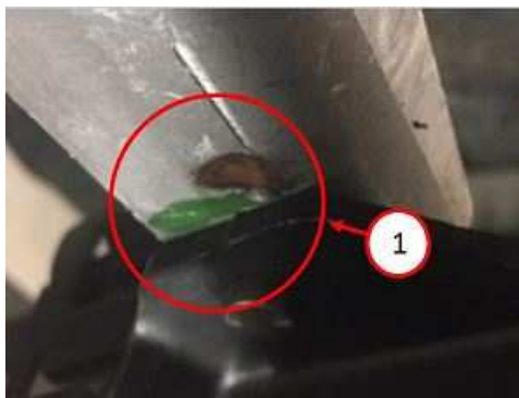
Fig. 2 Rust/Corrosion (Pivot Bracket)
