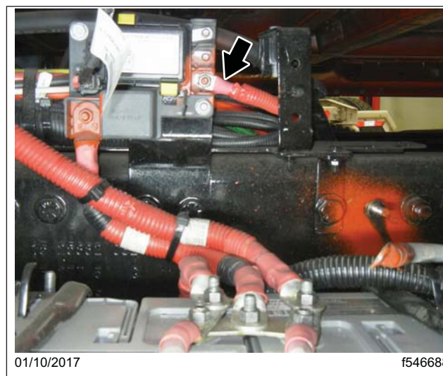
Fig. 28, CPDM Power Cable on the PNDB
